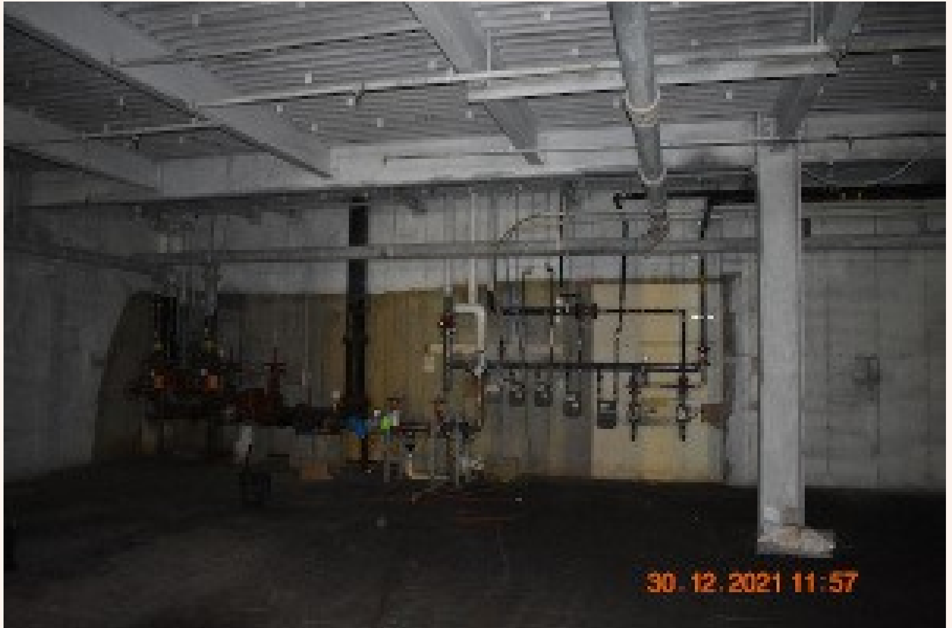
Open Basement area part of over 30,000 feet available This is the water wall. All water enters the building in this corner
