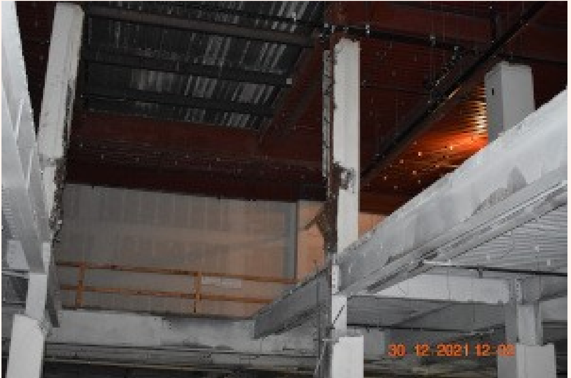
Open Basement area part of over 30,000 feet available This is where there was and escalator. The open hole is to be covered over.
