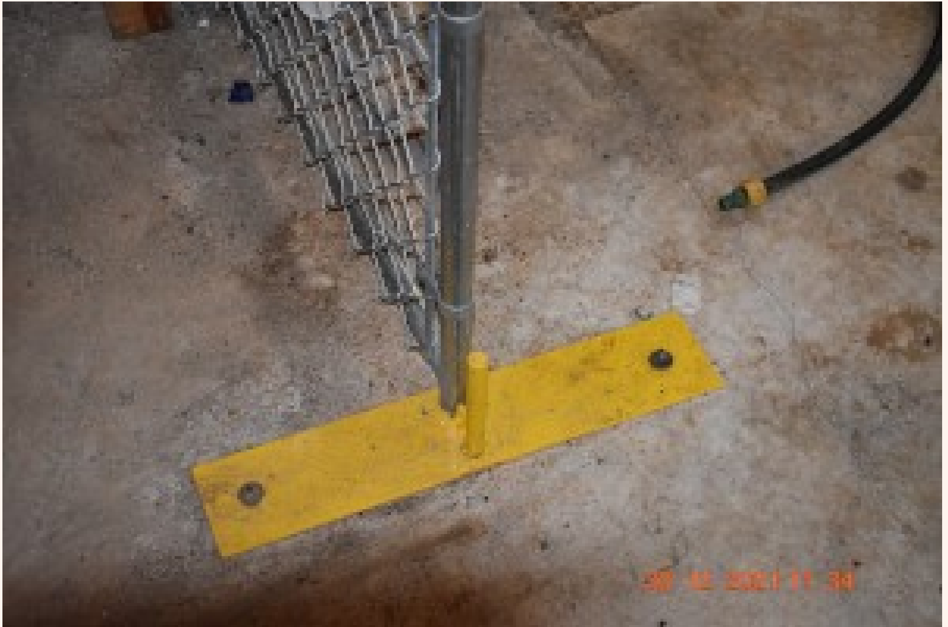
Star Tec Fenced in area Mounting plate on the floor for fence
