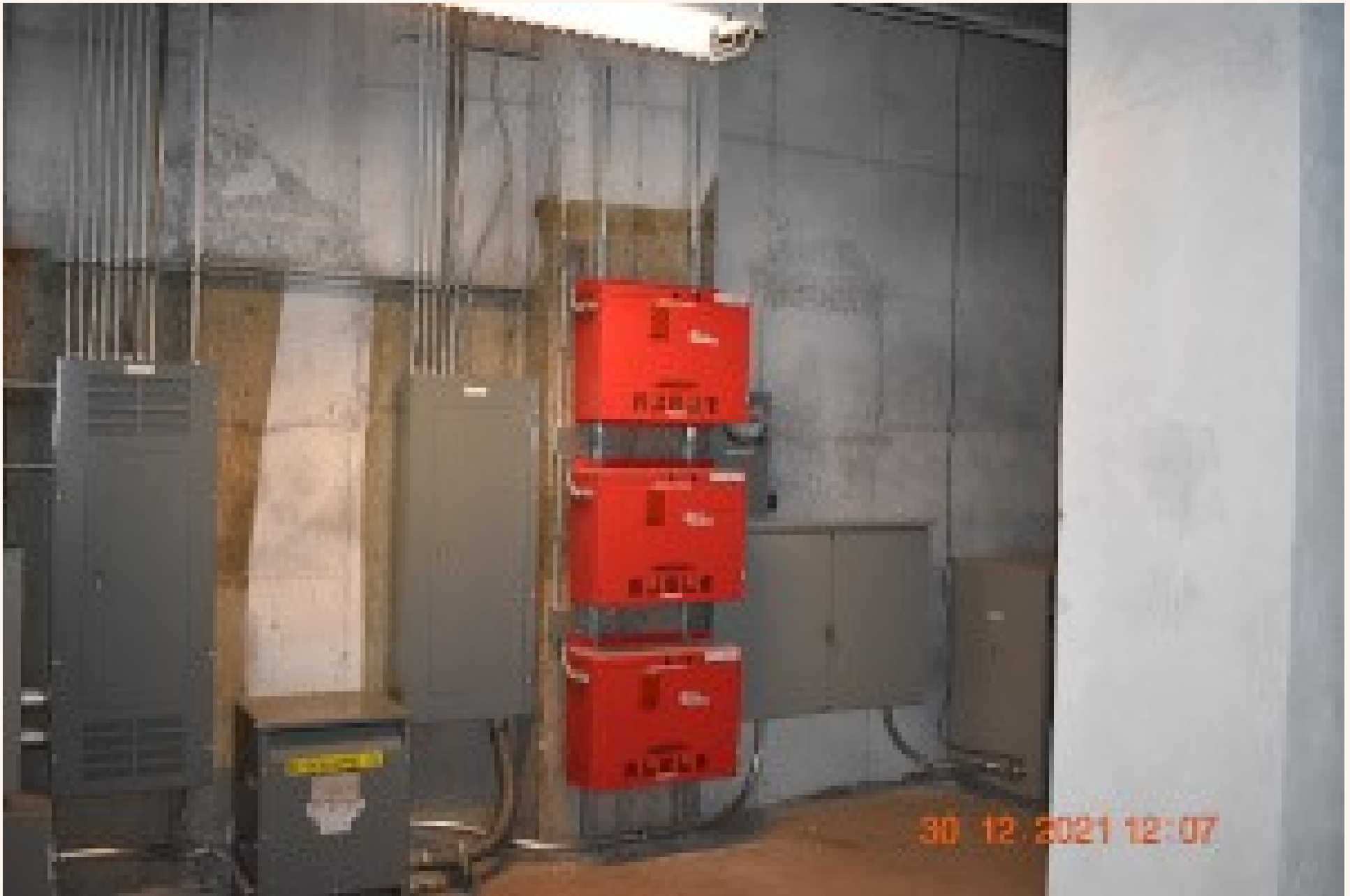
Open Basement area part of over 30,000 feet available Part of the Mechanical room with additional electric panels
