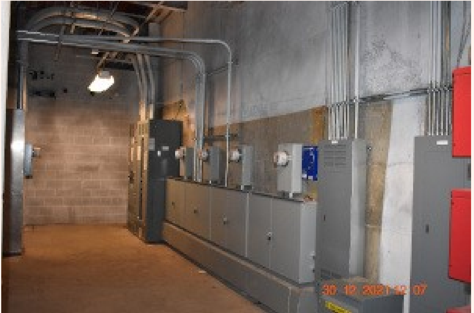
Open Basement area part of over 30,000 feet available Part of the Mechanical room with eclectic panels
