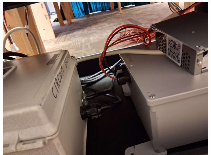
Bottom Shelf Transformer Cart
