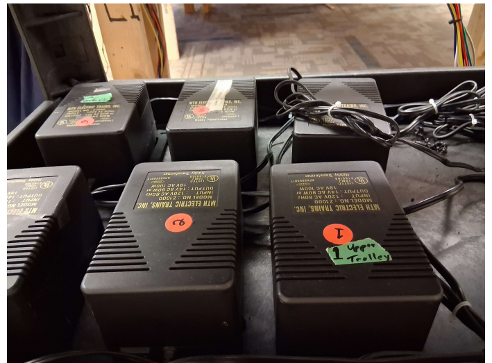
Center Shelf Transformer Cart
